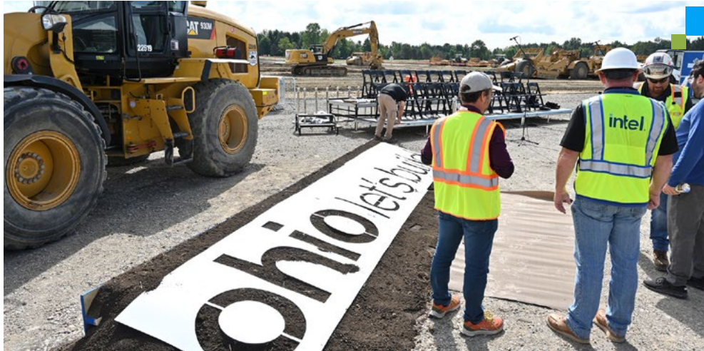
In September 2022, we celebrated our groundbreaking of two of the world’s most advanced chipmaking facilities, in Licking County, Ohio.
